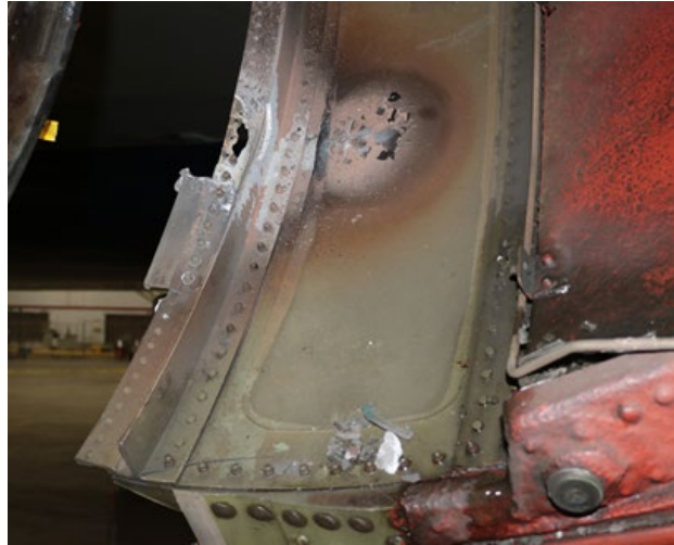
Figure 10. Inboard thrust reverser cowl thermal damage
