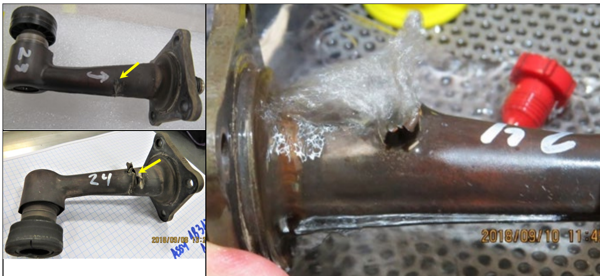
Figure 28. Mid-span impact damage to fuel nozzles 23 and 24 and leakage observed through stem of fuel nozzle 24
