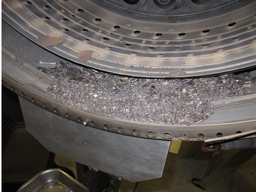
Photo No. 35: Close up view of the interior of the diffuser case showing small metal particles in the bottom of the case. (P&W)
