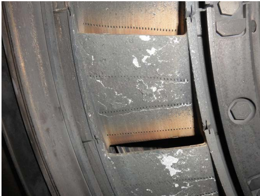
Photo No. 40: Close up view of 1st stage turbine vanes showing light coating of metal spray.
