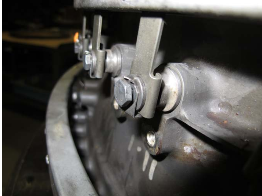
Photo No. 21: Close up view of a 5th stage VSV lever arm with the tab lock twisted out of position. (P&W)
