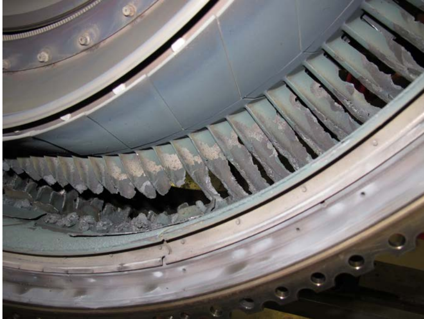
Photo No. 62: View of 3rd stage turbine vanes leading edges showing section burned out completely and other vanes partially burned away. (P&W)
