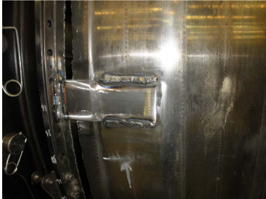
Photo No. 50: View of one of the metal plates that was welded onto the LPT case to facilitate removal of the LPT and turbine exhaust case from the HPT case.
