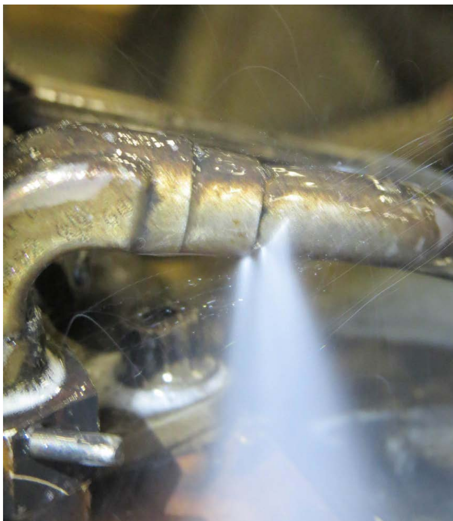
Photo 9- Manifold Supply Line Leak During Pressure Test
