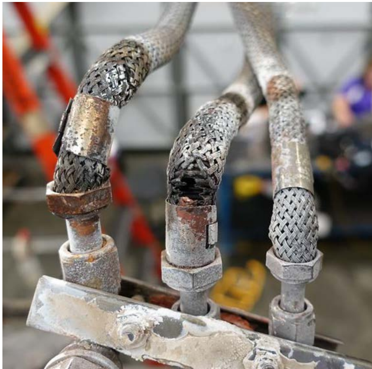
Photo 7- Pressure Regulating Line Thermal Damage, 12 o'clock as Viewed from the Right Side
