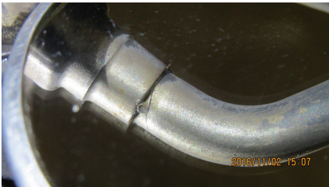
Photo 8- Manifold Supply Line Crack, 12 o'clock as Viewed With Inspection Mirror
