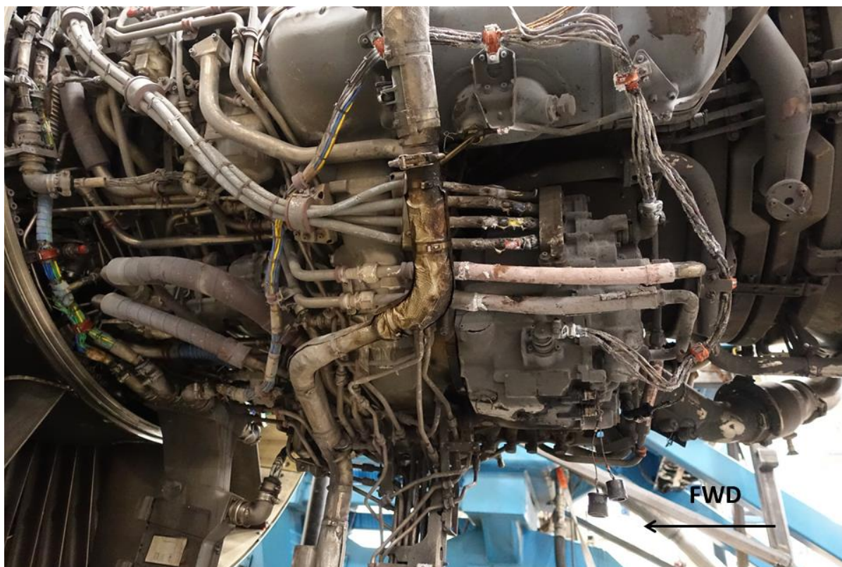
Photo 4- Soot/Discoloration and Thermal, 6 to 9 o'clock
