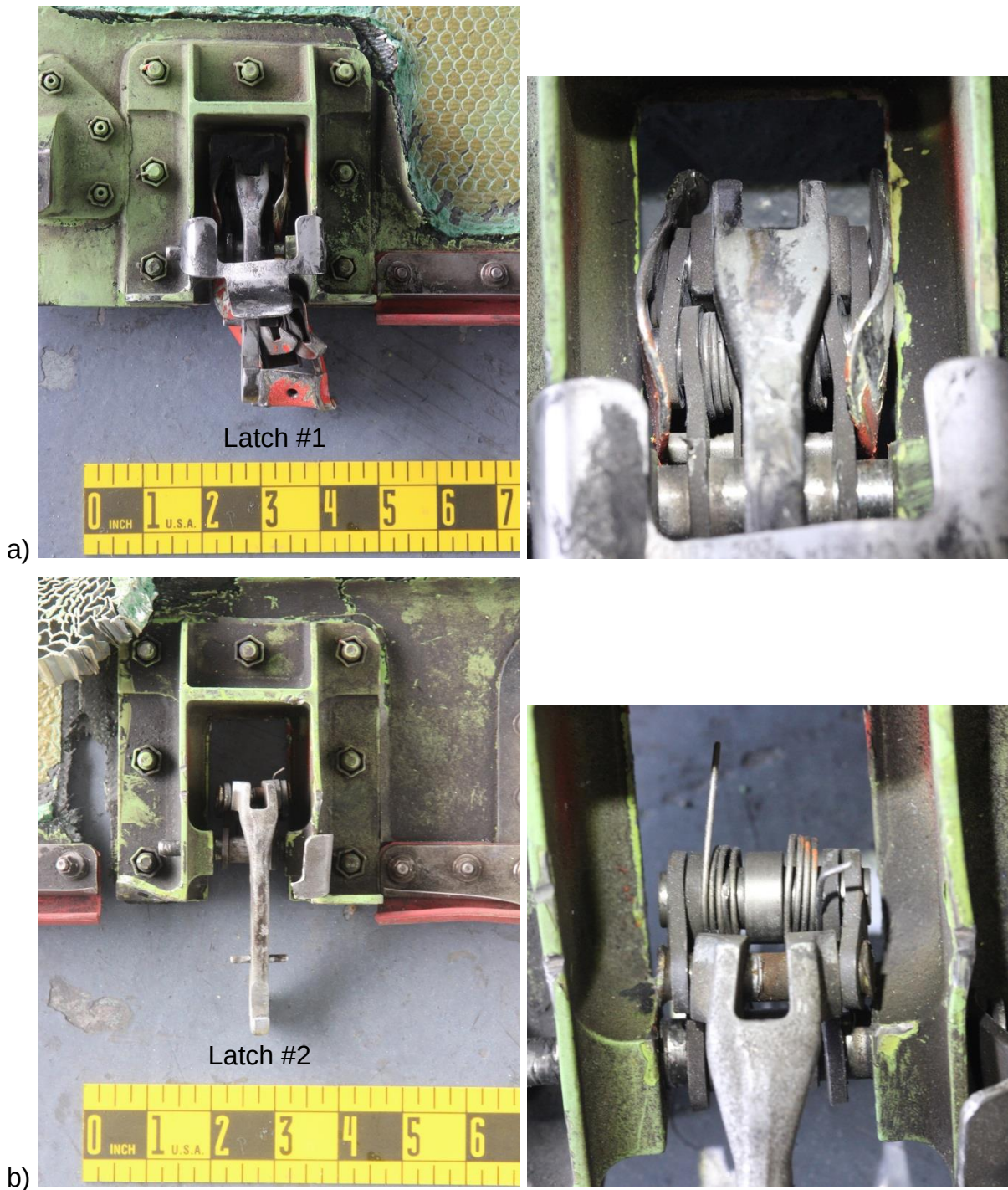
Figure 6: Photos of the fan cowl handles/latches and link mechanisms. Latches are numbered 1 through 4 starting at the forward end of the cowl; a) latch #1; b) latch #2;
