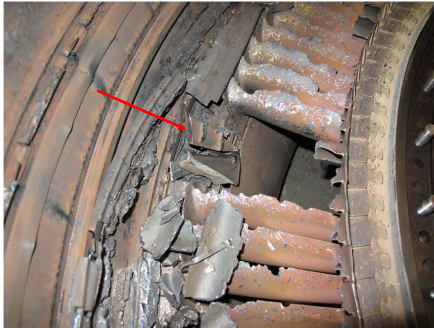
Photo No. 3: View from the rear of the location of the missing 3rd stage vane cluster with an arrow pointing to the piece of 3 rd stage vane cluster inner shroud. (P&W)
