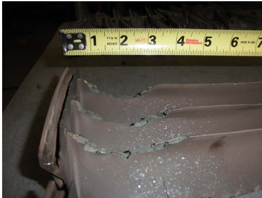
Photo No. 22: Close up view showing damage to 6th stage turbine vane cluster airfoil leading edges.
