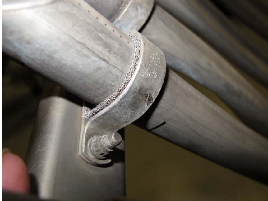
Photo No. 25: Close-up view of dent on turbine cooling air manifold clamp. (P&W)
