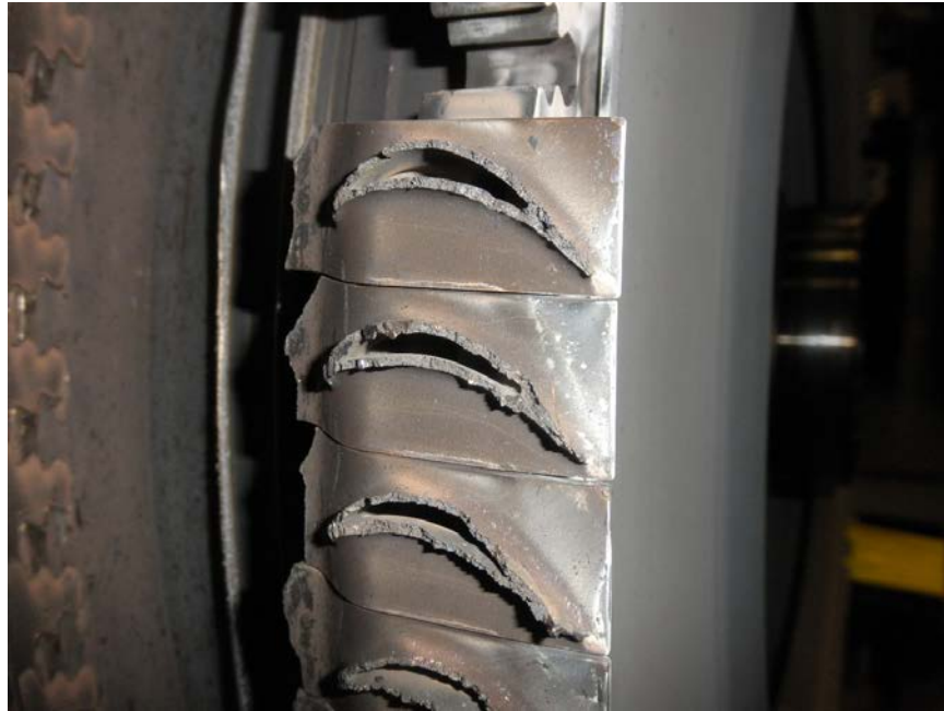
Photo No. 24: Close-up view of 5th stage turbine blades showing coarse and grainy fracture surfaces.
