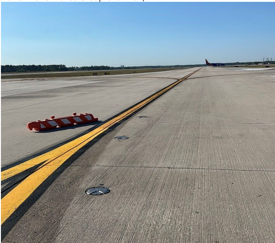
Figure 8: Displaced Construction Barricade (Postincident) on Taxiway H. Incident Airplane in Background (Source: Greater Orlando Airport Authority)
