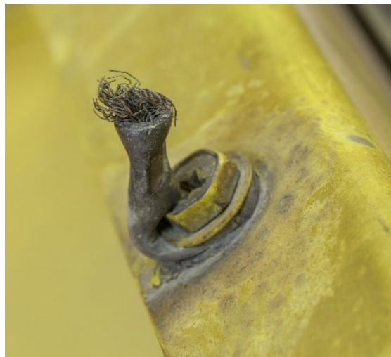
Figure 14: Broken bonding strap
