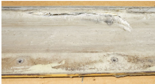
Figure 87: Damage on inner surface of panel seal
