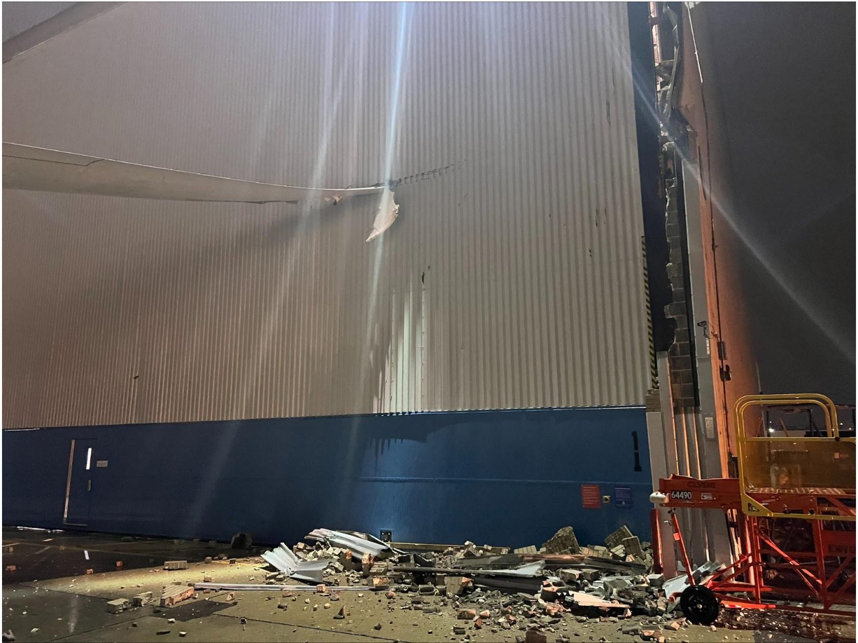
Photo 2 – Damaged aircraft hangar.
