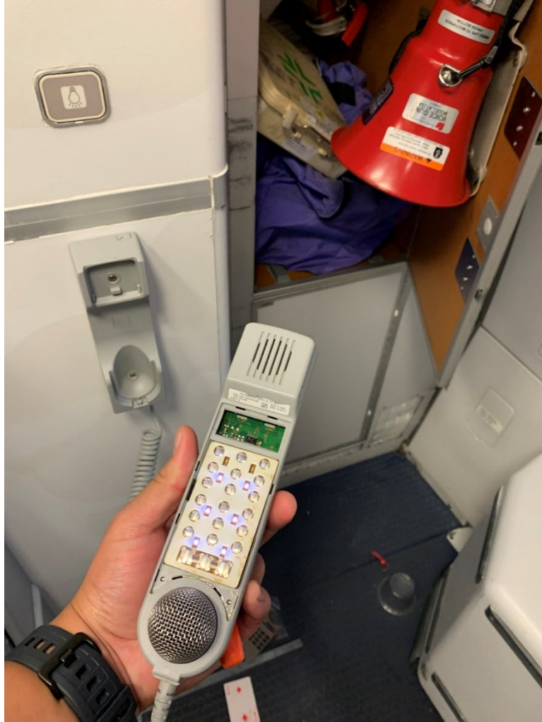
Figure 5. Damaged 4L flight attendant handset.
