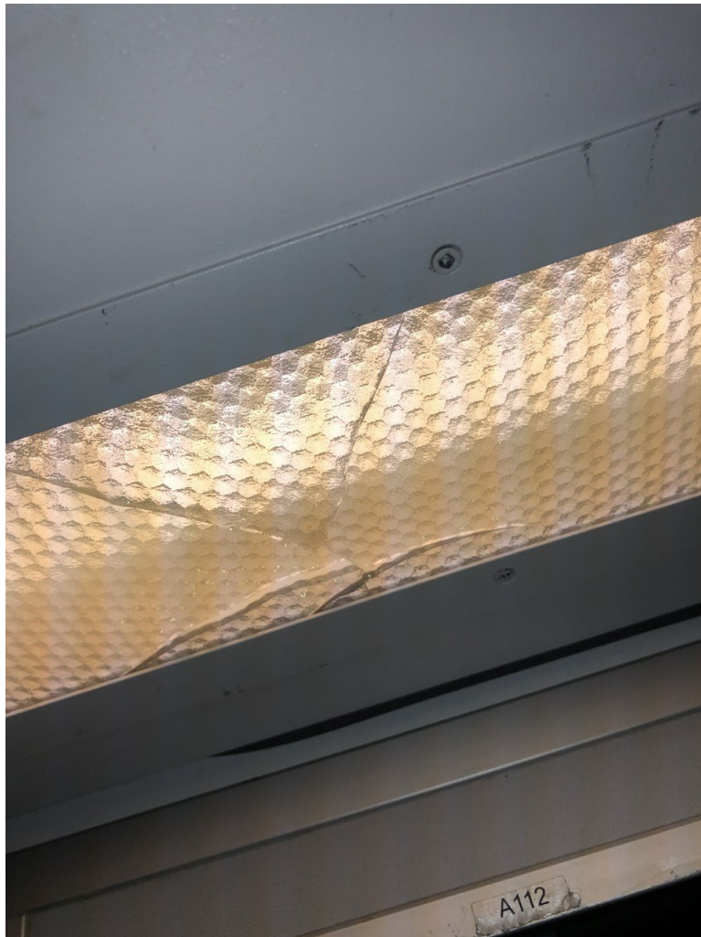
Figure 4. Crack in an overhead light in the rear galley area.
