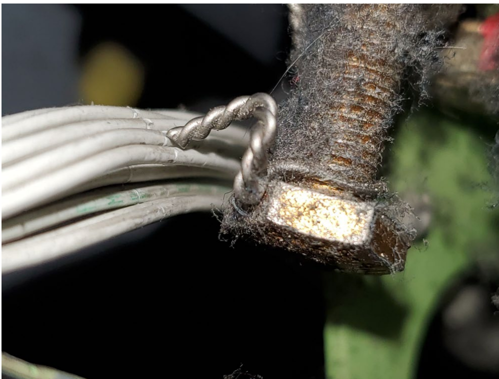
Figure 3: Incorrectly Tucked Safety Wire Contacting Electrical Wires
