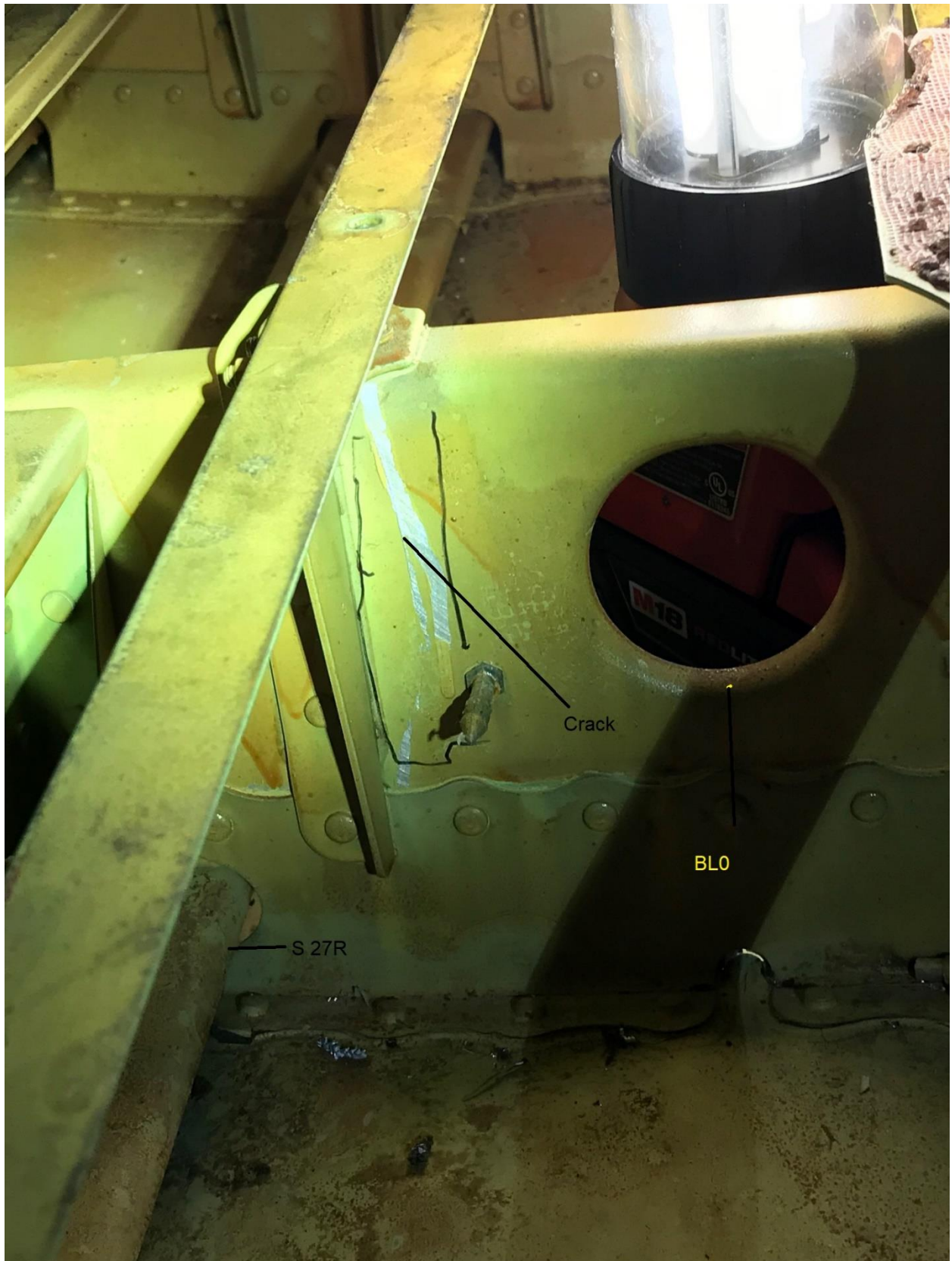
Figure 4-5 STA 867 Frame crack
