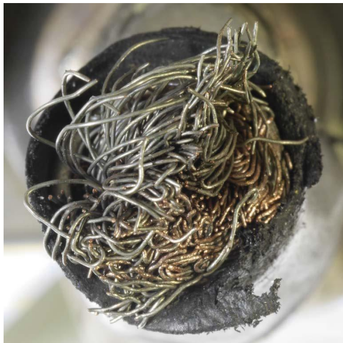
Figure 8: Fractured ground wire termination point
