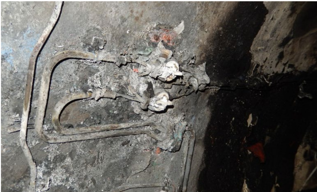
Photo 23- No. 2 Engine Right (Outboard) Thrust Reverser Door, Fire Detection System Damage
