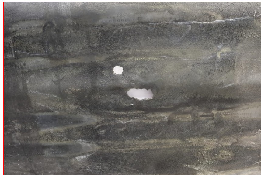
Dark, mottled surface with sooting and metal splatter
