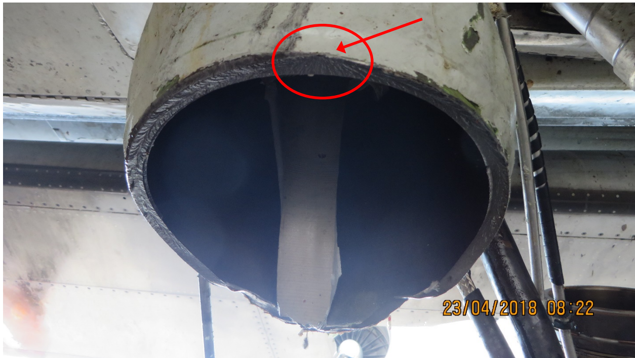
Figure 6 - Upper cylinder fatigue crack initiation site (forward side).
