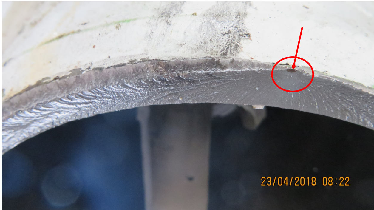
Figure 7 – Upper cylinder fatigue crack initiation site (forward side).
