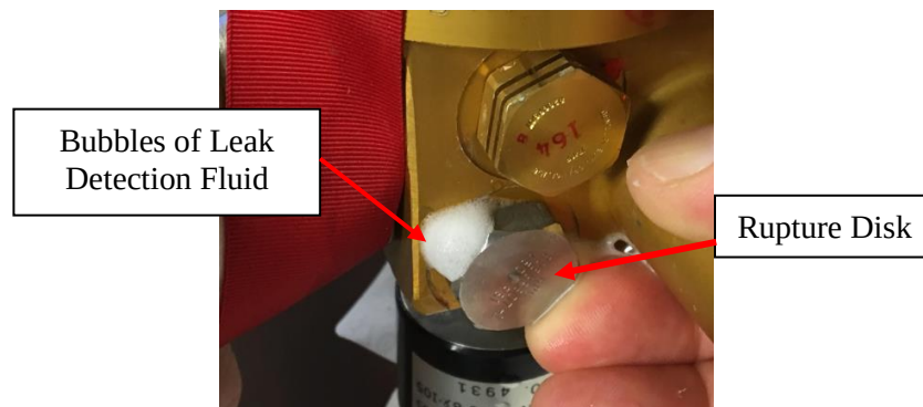
Figure 11 Rupture Disk Outlet Leaking
