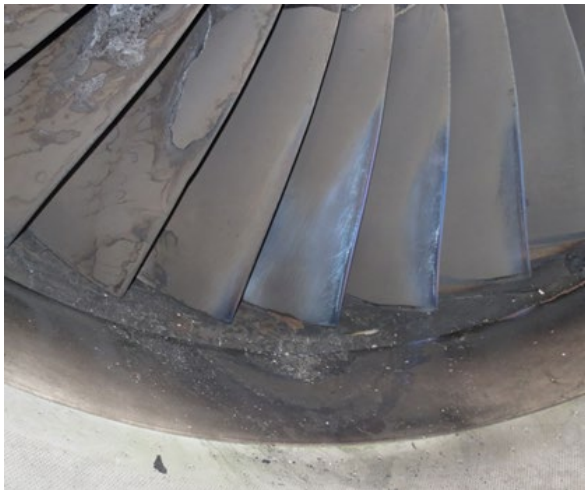
Figure 17. Fan blade and blade path thermal damage
