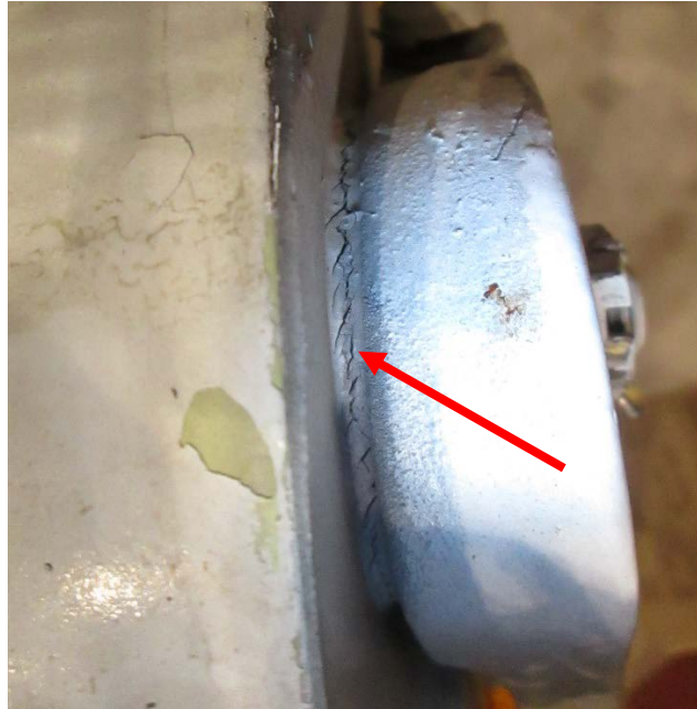
Figure 22 - Sealant (cracking noted by arrow) between the LH elevator stop arm and closeout rib.
