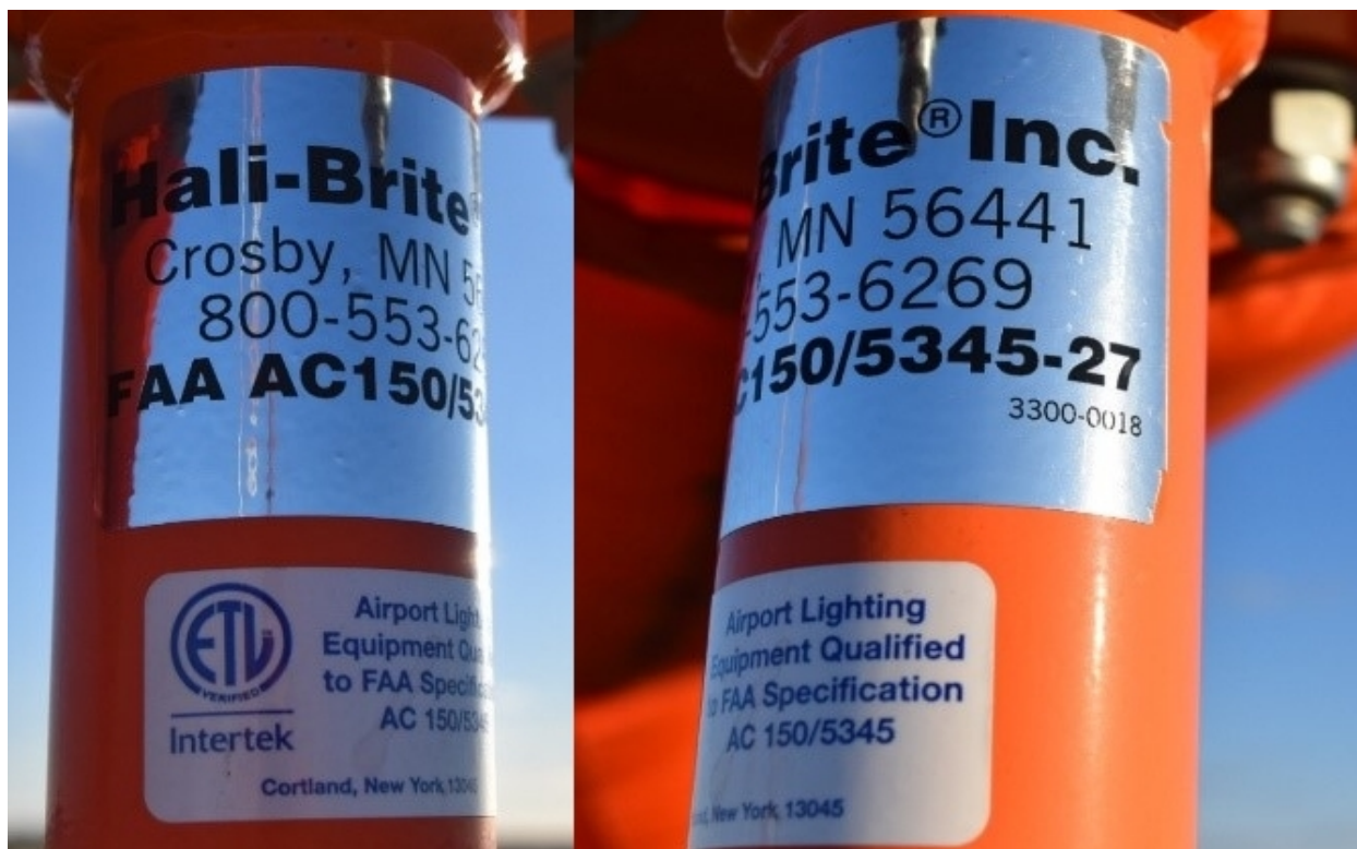
Figure 9 – Manufacturer’s stickers located on the YIP Runway 23L Approach supplemental windsock pole.
