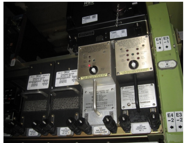
PHOTO 56: BUS POWER CONTROL UNIT WITH FAULT LIGHT ILLUMINATED
