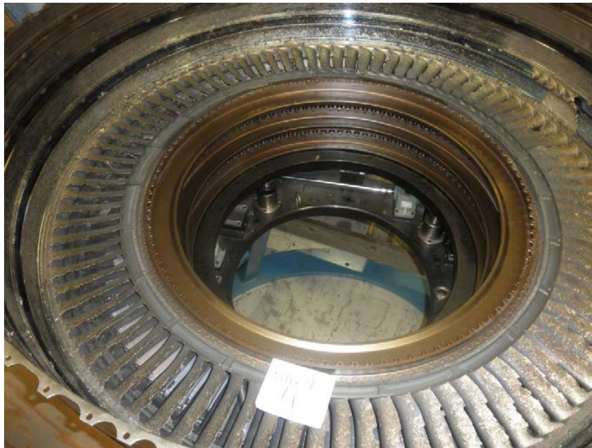
Photo No. 28: View of LPT stage 4 nozzles showing all are in place. Also shown are the LPT stage 4 shroud segments showing all are missing except one and the LPT stage 5 nozzles showing that all are missing except one platform hook.
