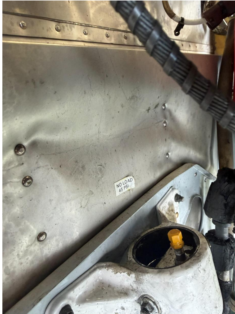
Photograph 1 - Firewall Substantial Damage (Courtesy of Operator)
