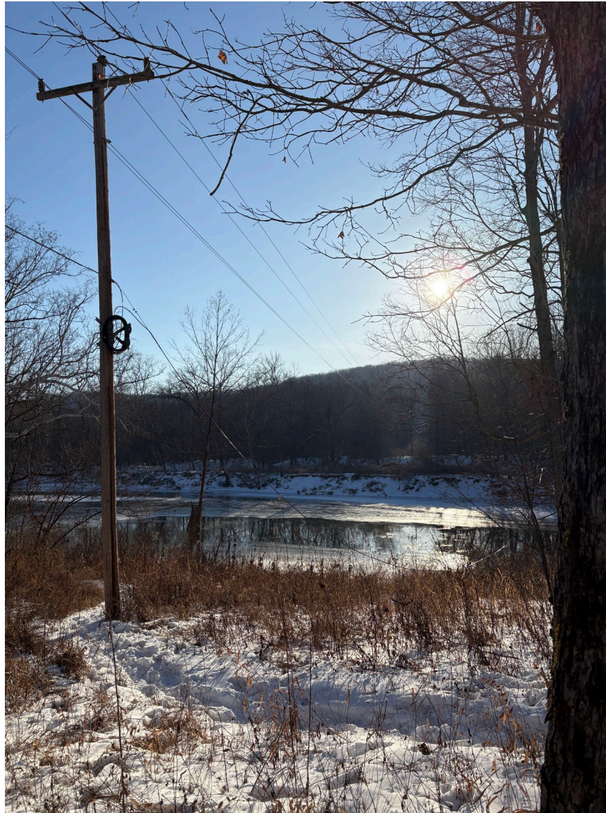
Photograph 1 - Downed Powerline (Courtesy of FAA)
