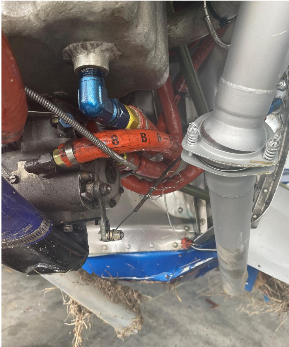
Photograph 5 - Mixture linkage with severed safety wire (Courtesy of NTSB)
