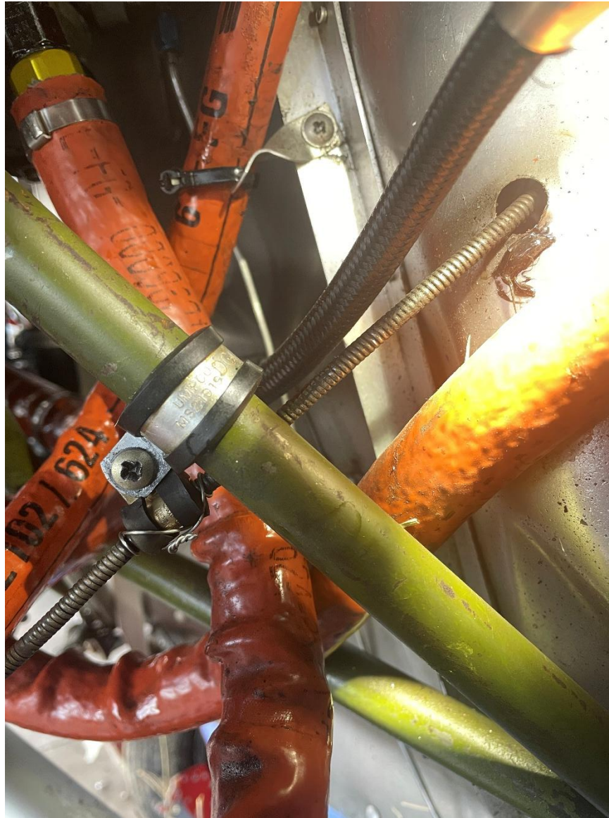
Photograph 7 - Mixture cable slippage (Courtesy of NTSB)
