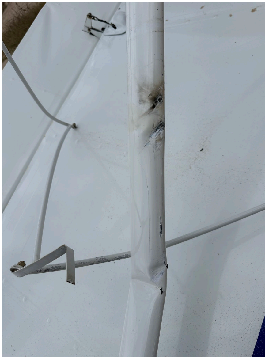
Photograph 5 - Bent wing strut (Courtesy of FAA)
