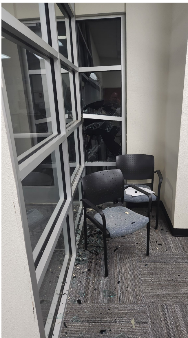
Photograph 5 - Terminal Building Damage (Courtesy of Airport Manager)
