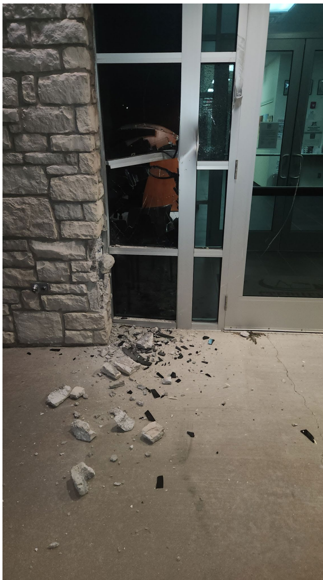
Photograph 4 - Terminal Building Damage (Courtesy of Airport Manager)
