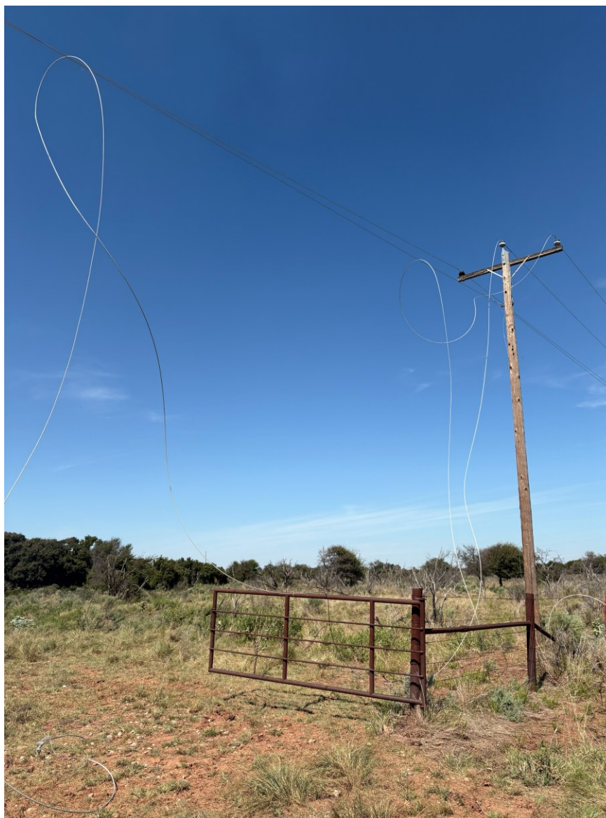
Photograph 2 - Powerline damage (Courtesy of pilot)
