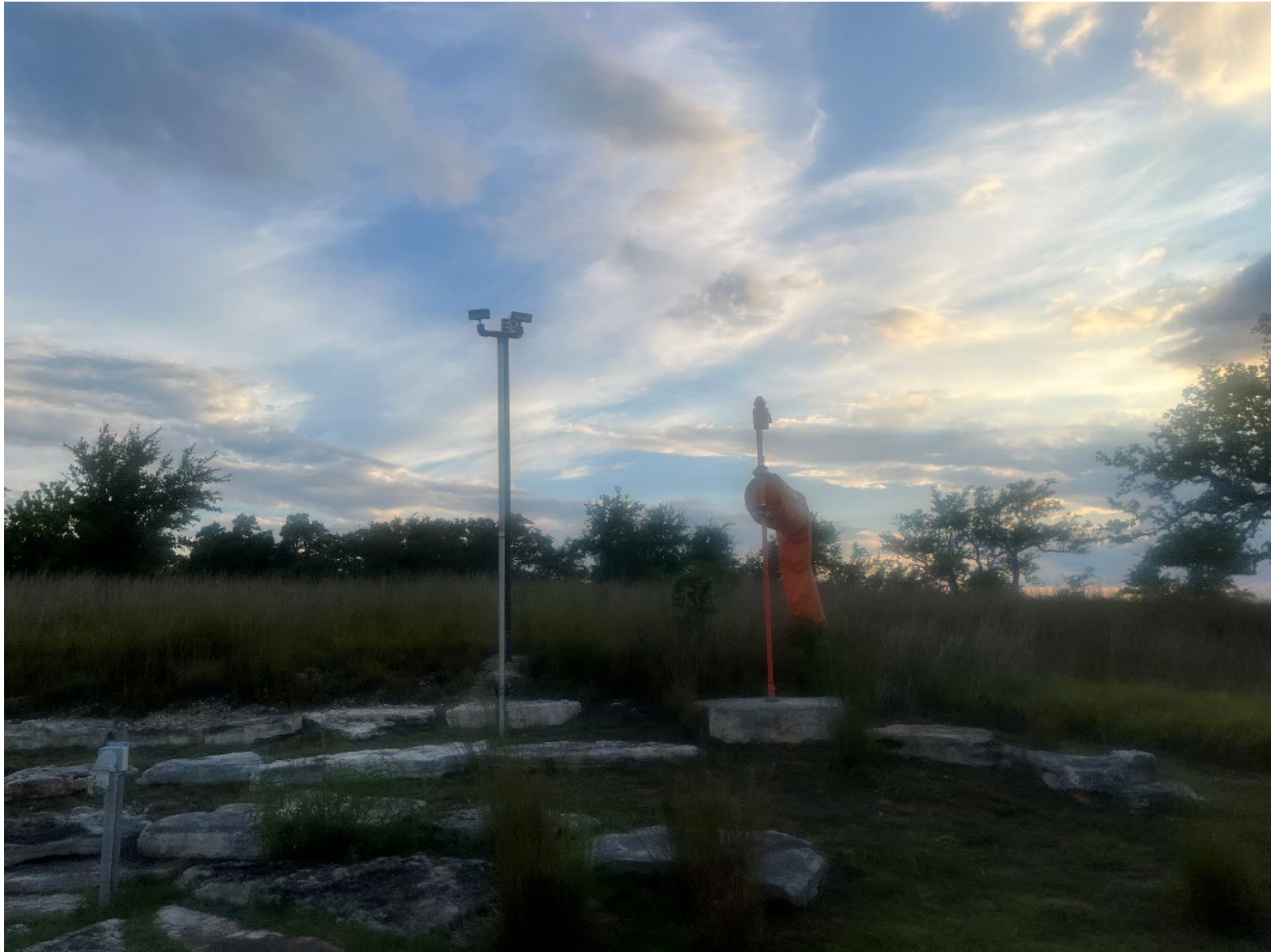
Photograph 9 - View of the private heliport lighting and lighted wind cone (courtesy of the Federal Aviation Administration)
