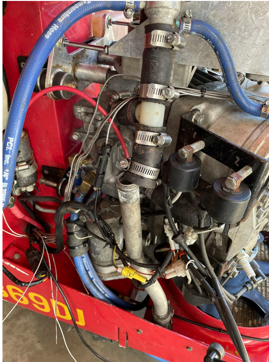
Photograph 3 - Engine Coolant Hose (NTSB Photo)
