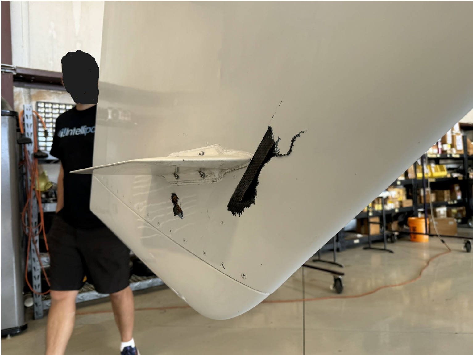
Photograph 1 - Ventral Stabilizer Damage (Courtesy of Addison Airport Manager)
