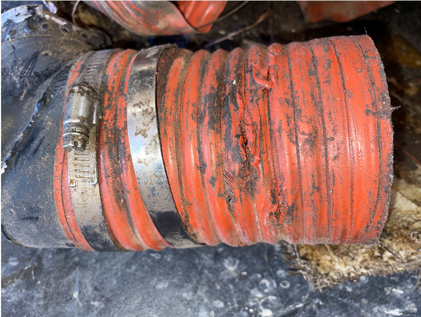
Photograph 13 - Scat duct holes and repairs (Courtesy of NTSB)
