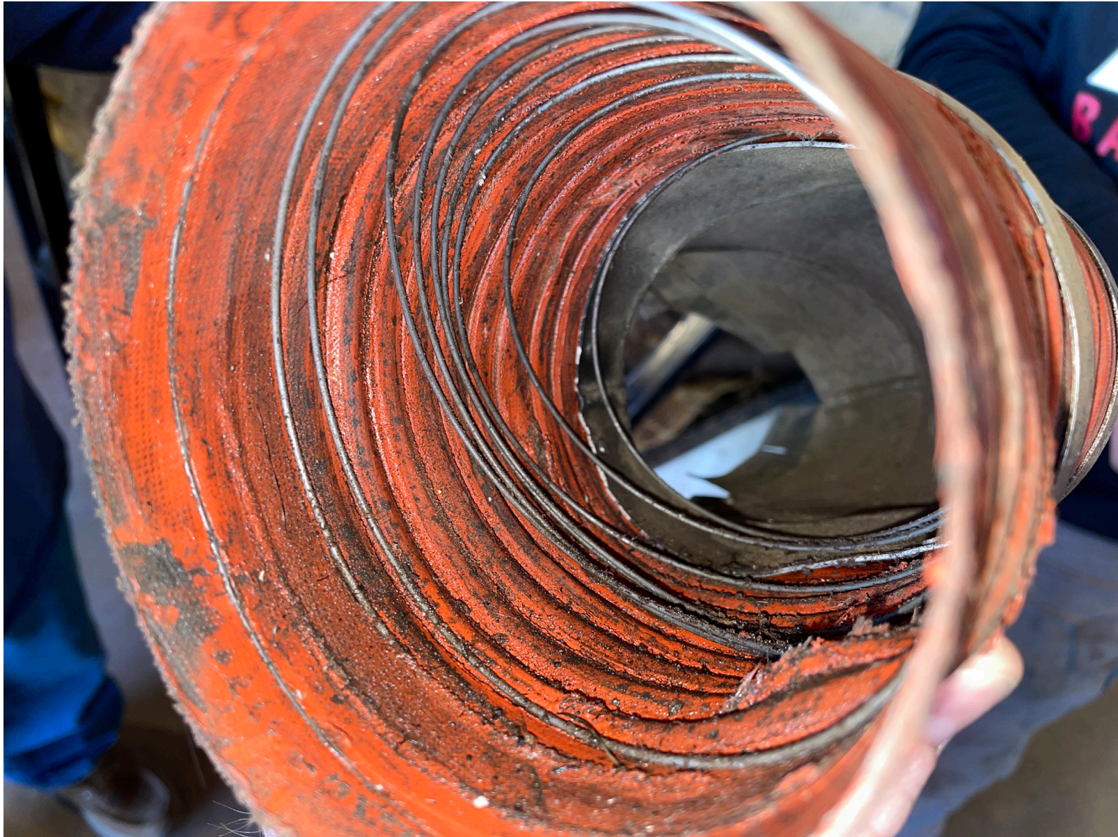
Photograph 9 - Collapsed and degraded scat duct (Courtesy of NTSB)
