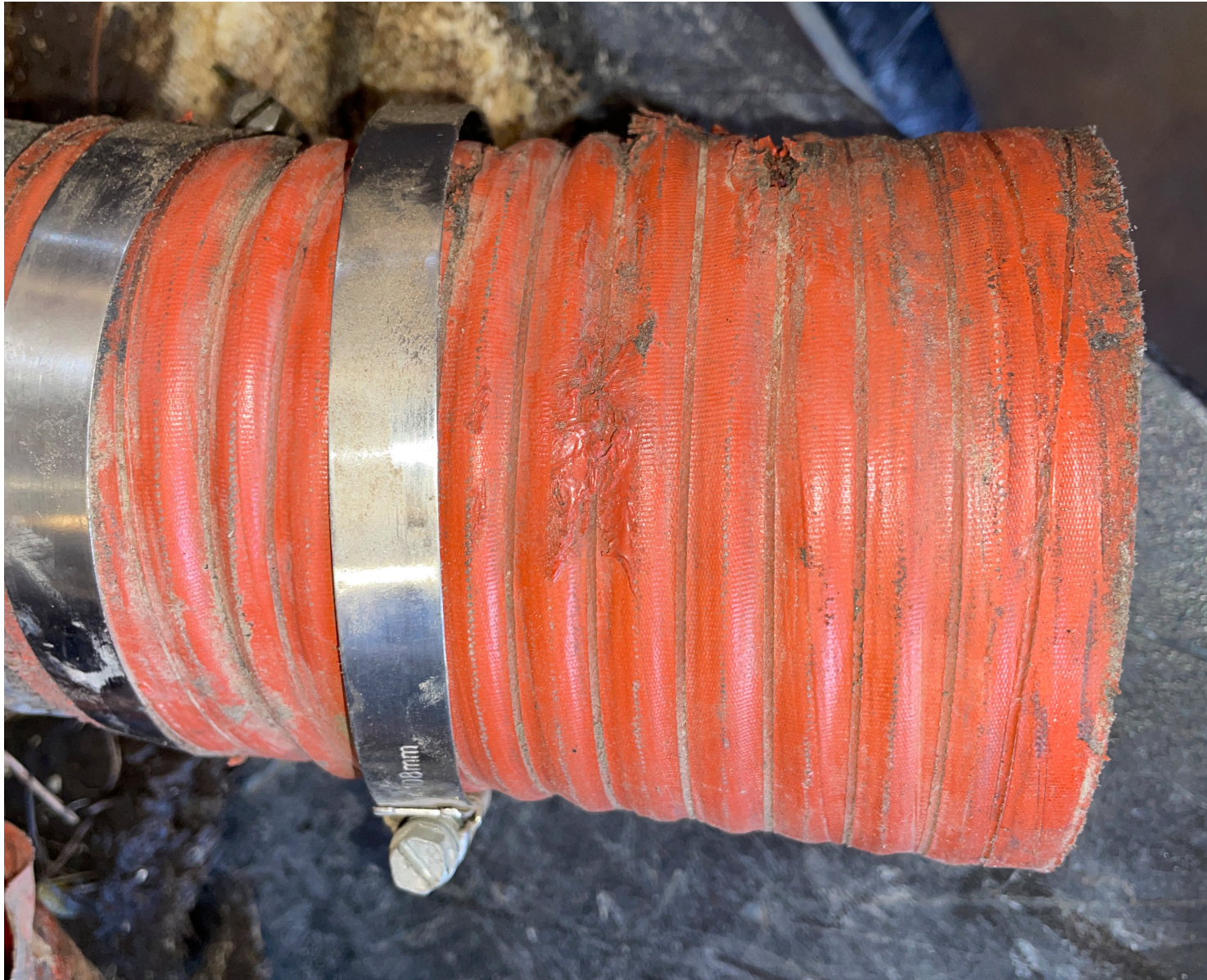
Photograph 12 - Scat duct holes and repairs (Courtesy of NTSB)
