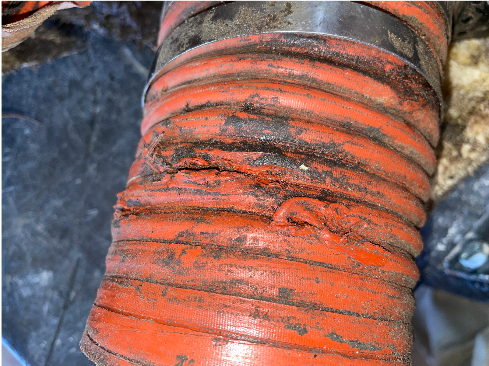
Photograph 11 - Scat duct holes and repairs (Courtesy of NTSB)
