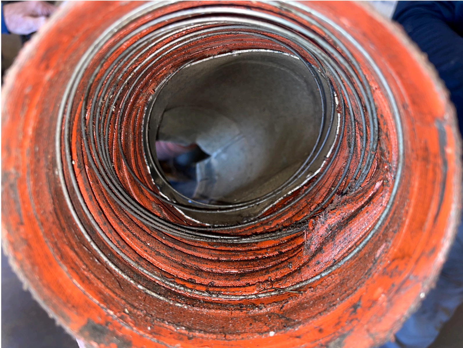
Photograph 10 - Collapsed and degraded scat duct (Courtesy of NTSB)
