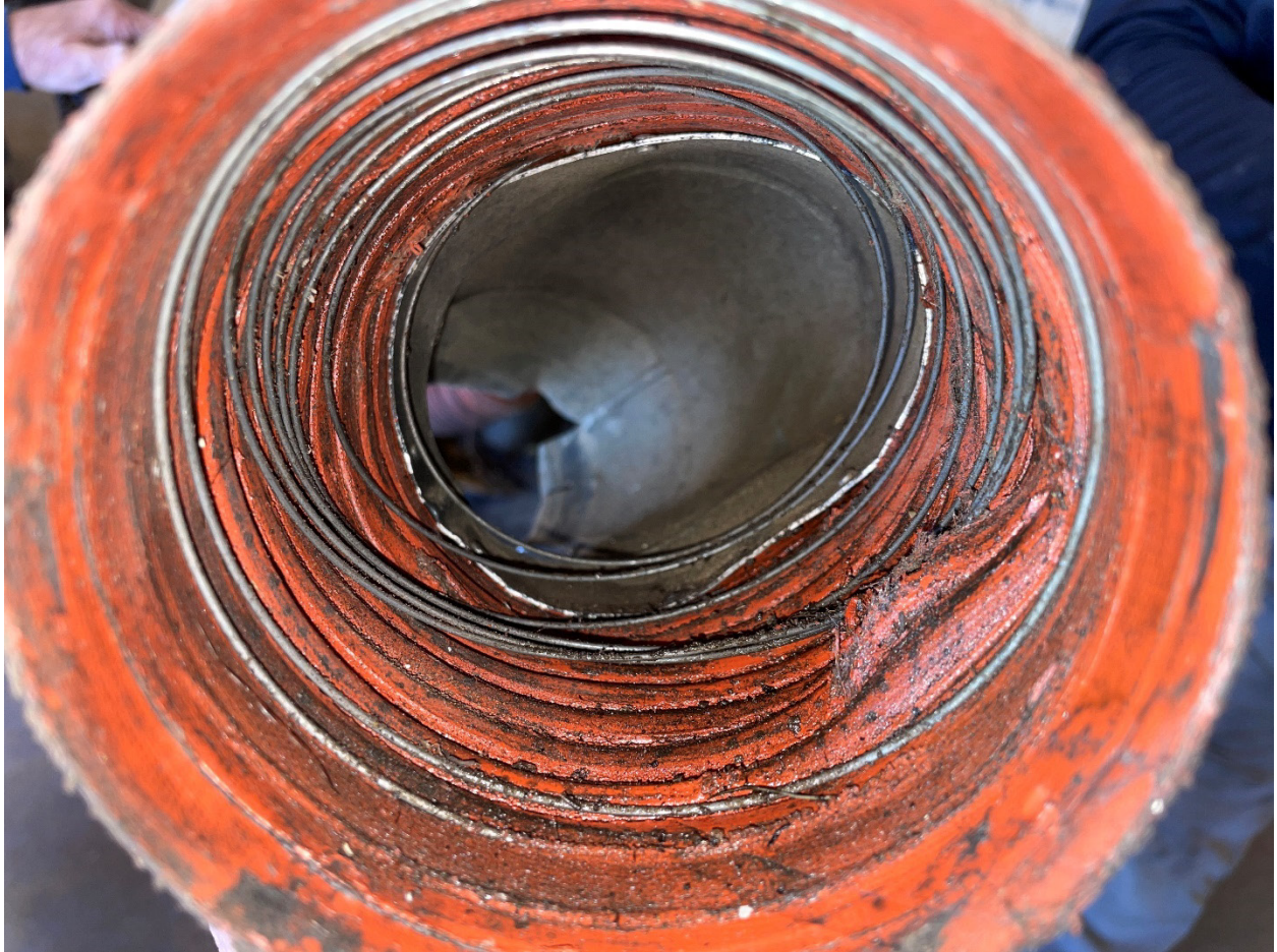
Figure 1. Inside view of the failed scat duct.
