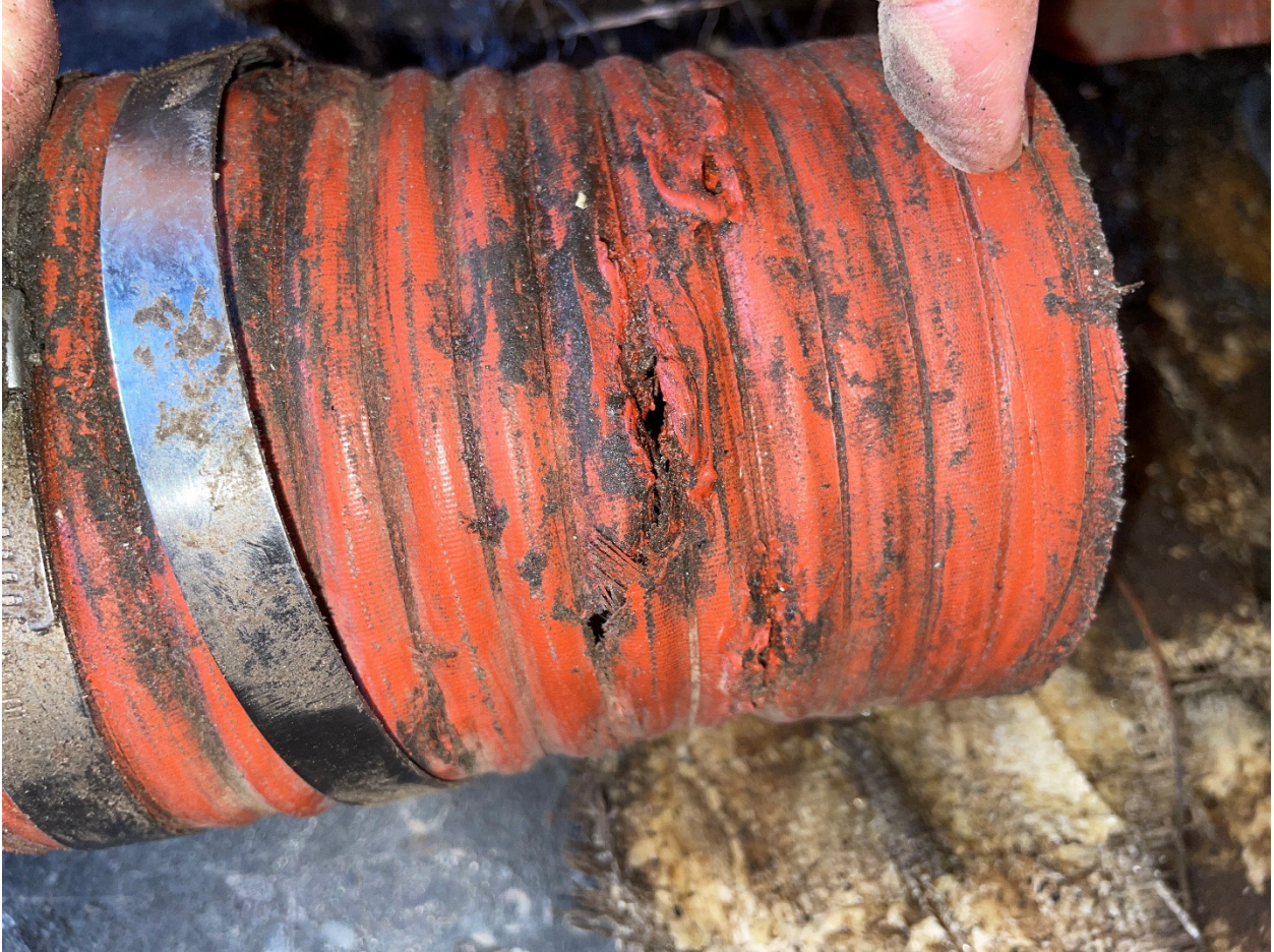
Figure 2. Outside view of the failed scot duct with several holes and orange silicone on and near the holes.
