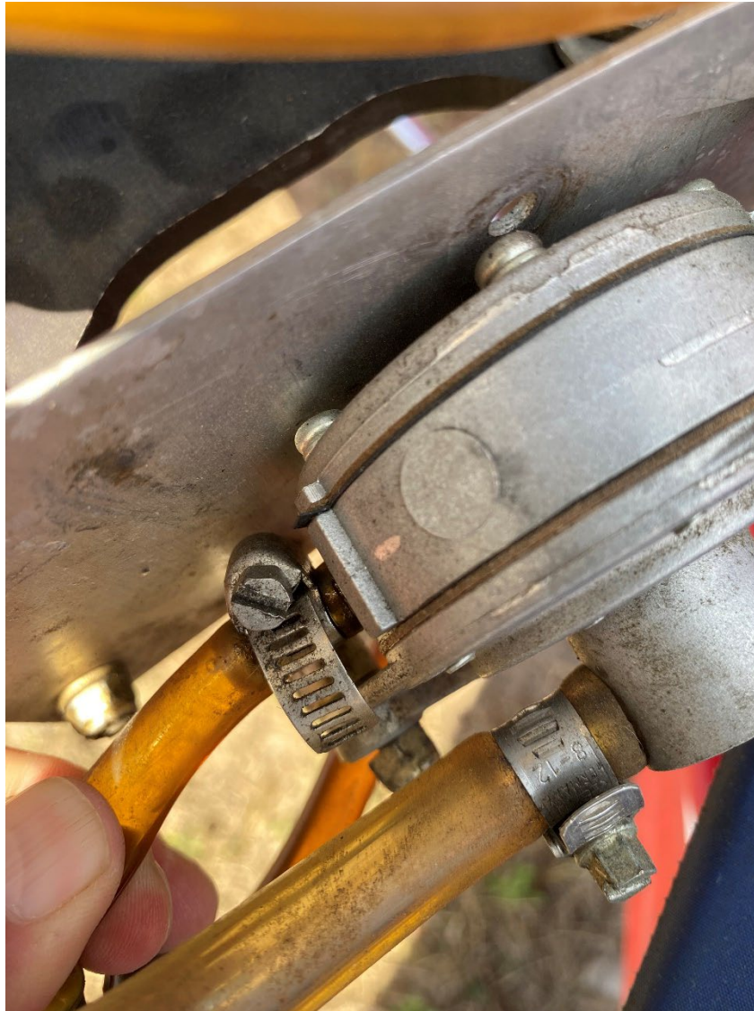
Photograph 2 - Fuel pump fuel line (Source: Federal Aviation Administration).
