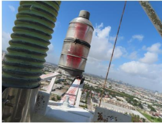
Figure 11. Image of one of the beacons attached to the radio tower. Photo courtesy of the owner.
