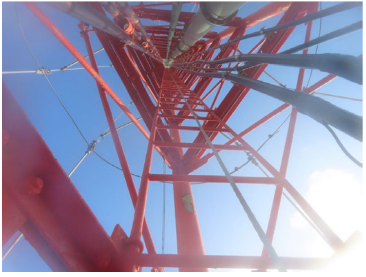
Climbing Facilities on Leg A
