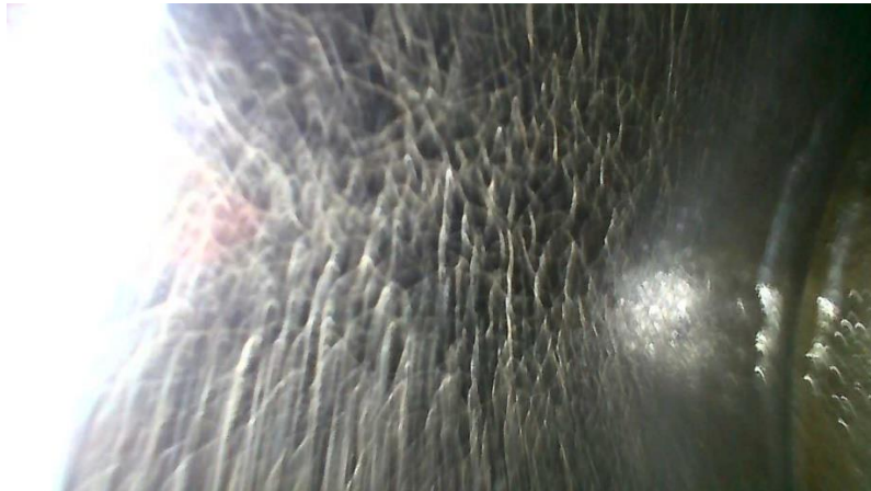
Crackling in Cylinder wall, found in all cylinders
