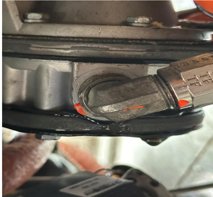
Engine Driven Fuel Pump Fitting with Loose Jam Nut
