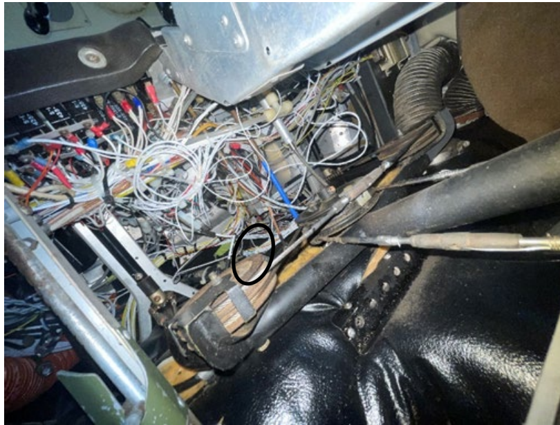
Figure 2 - Instrument Panel Wiring with Wire Chaffing (Shown in the Black Circle)
