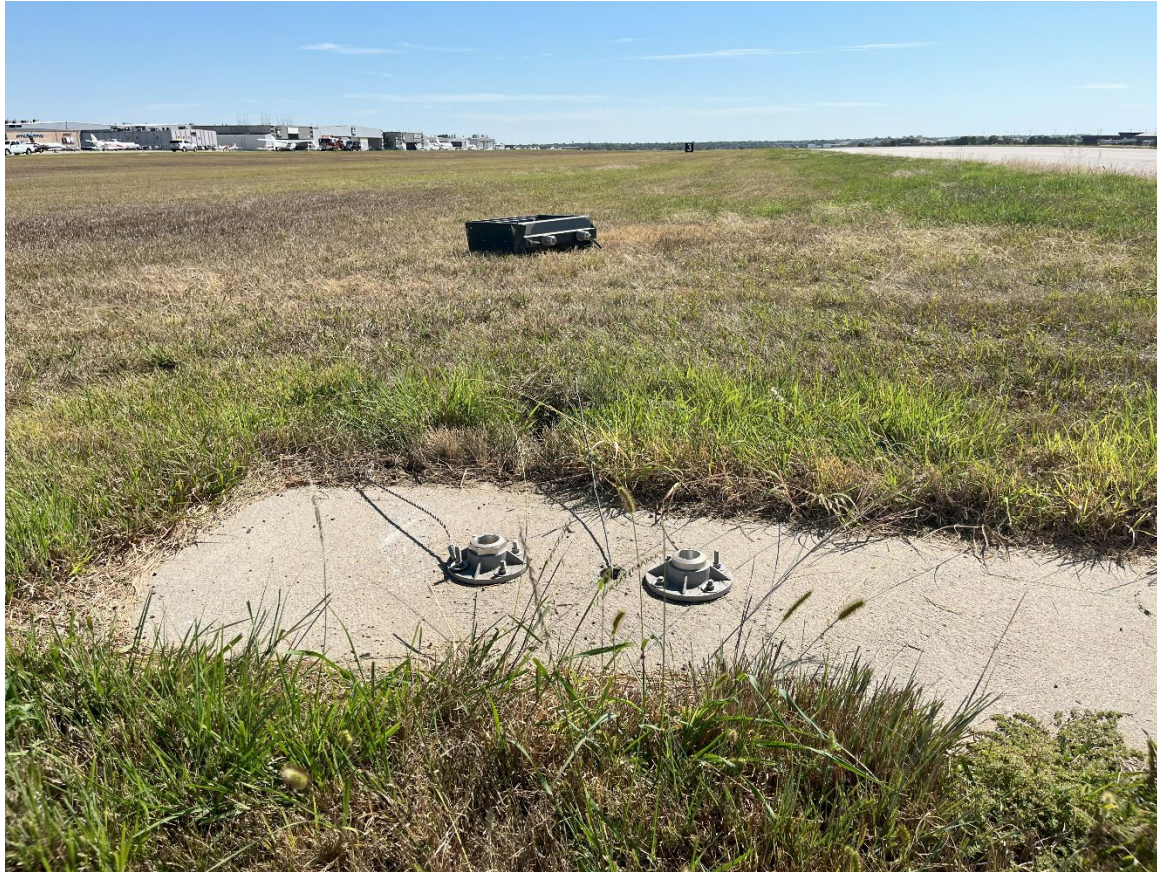
Photograph 3 - Damaged runway sign (FAA Photo)
