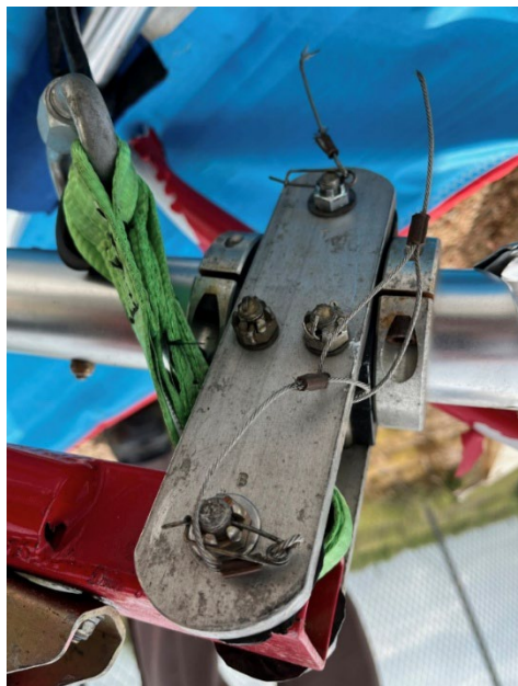
Figure 3. Hang Point Nuts and Bolts (Provided by FAA)
