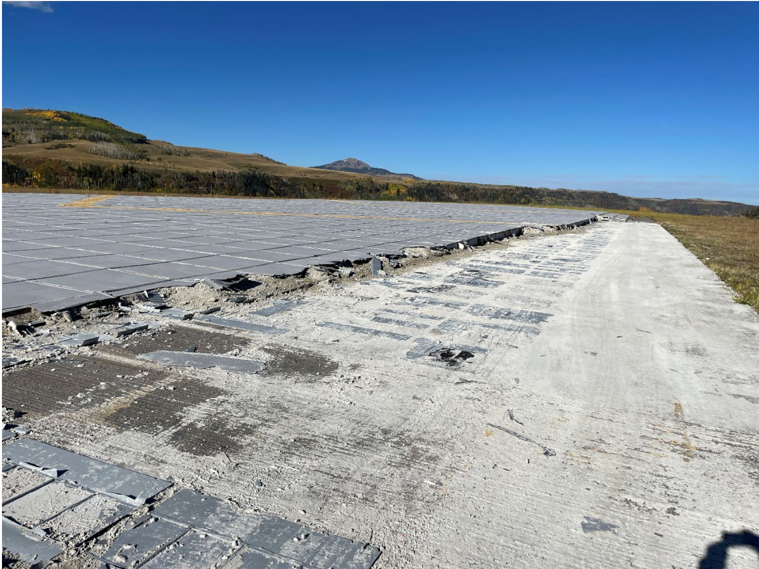
Photograph 5 - West facing view of the damage sustained to the engineered material arresting system from the airplane
