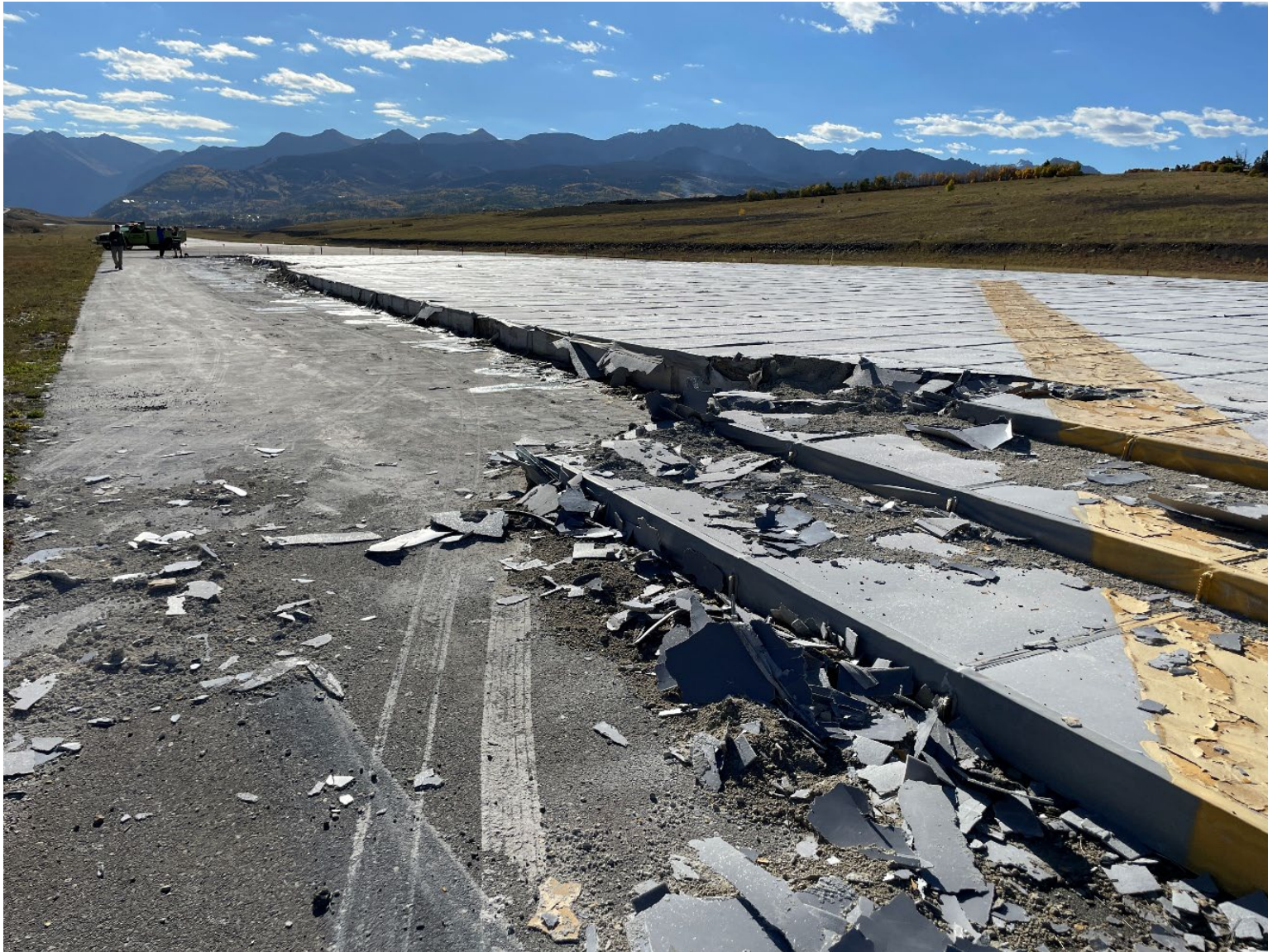
Photograph 4 - East facing view of the damage sustained to the engineered material arresting system from the airplane
