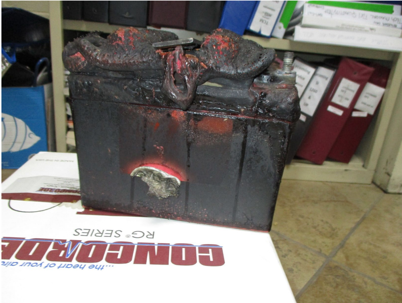
Photograph 5: Damage to Battery (Courtesy of the Federal Aviation Administration)
