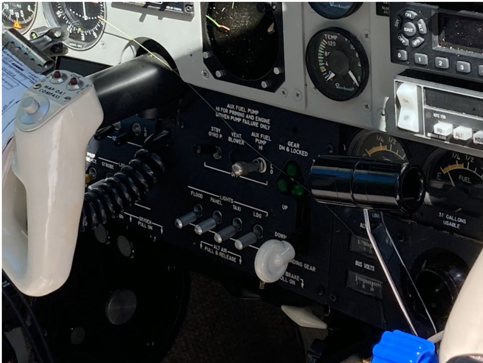
Photograph 2 - Auxiliary Fuel Pump (Courtesy of FAA)
