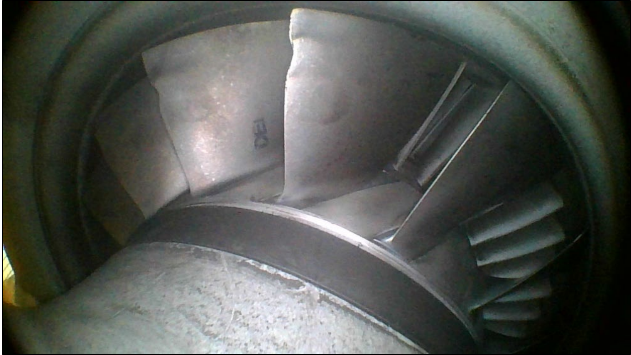
Figure 21: View of stage 1 compressor blade leading edges
