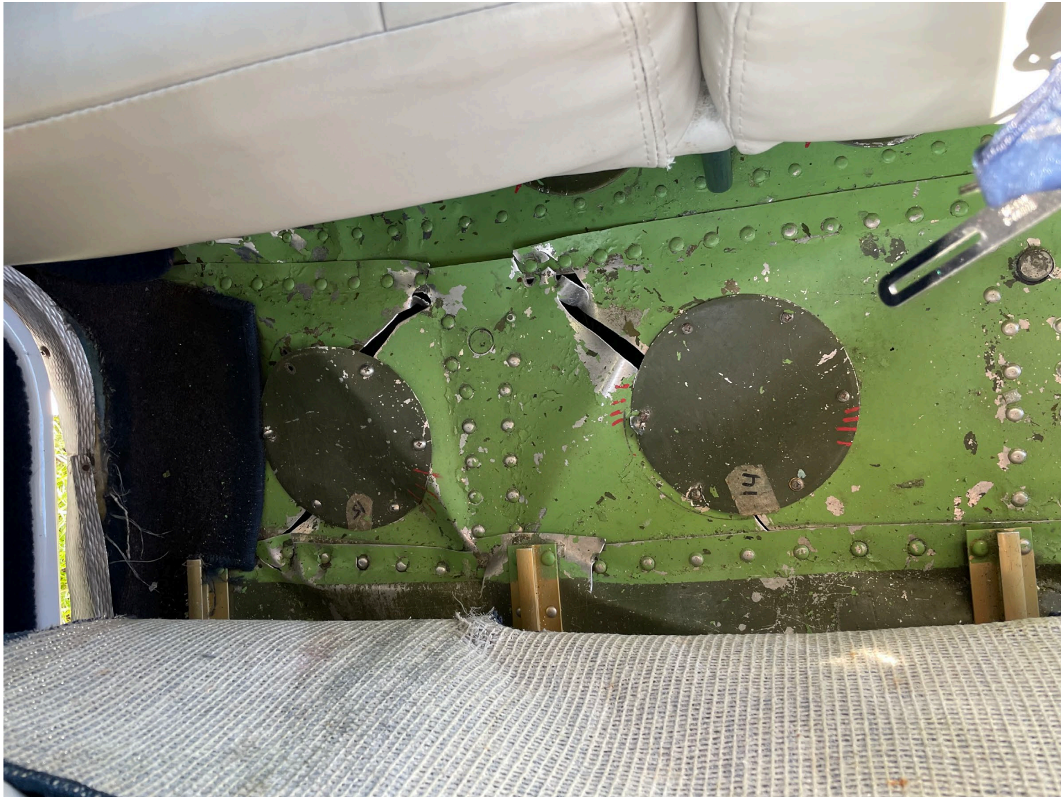
Photograph 4 - Interior Fuselage Damage (Courtesy of FAA)
