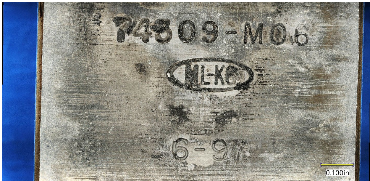
Figure 32. Exterior of the C4 bearing, showing the part numbers and markings.
