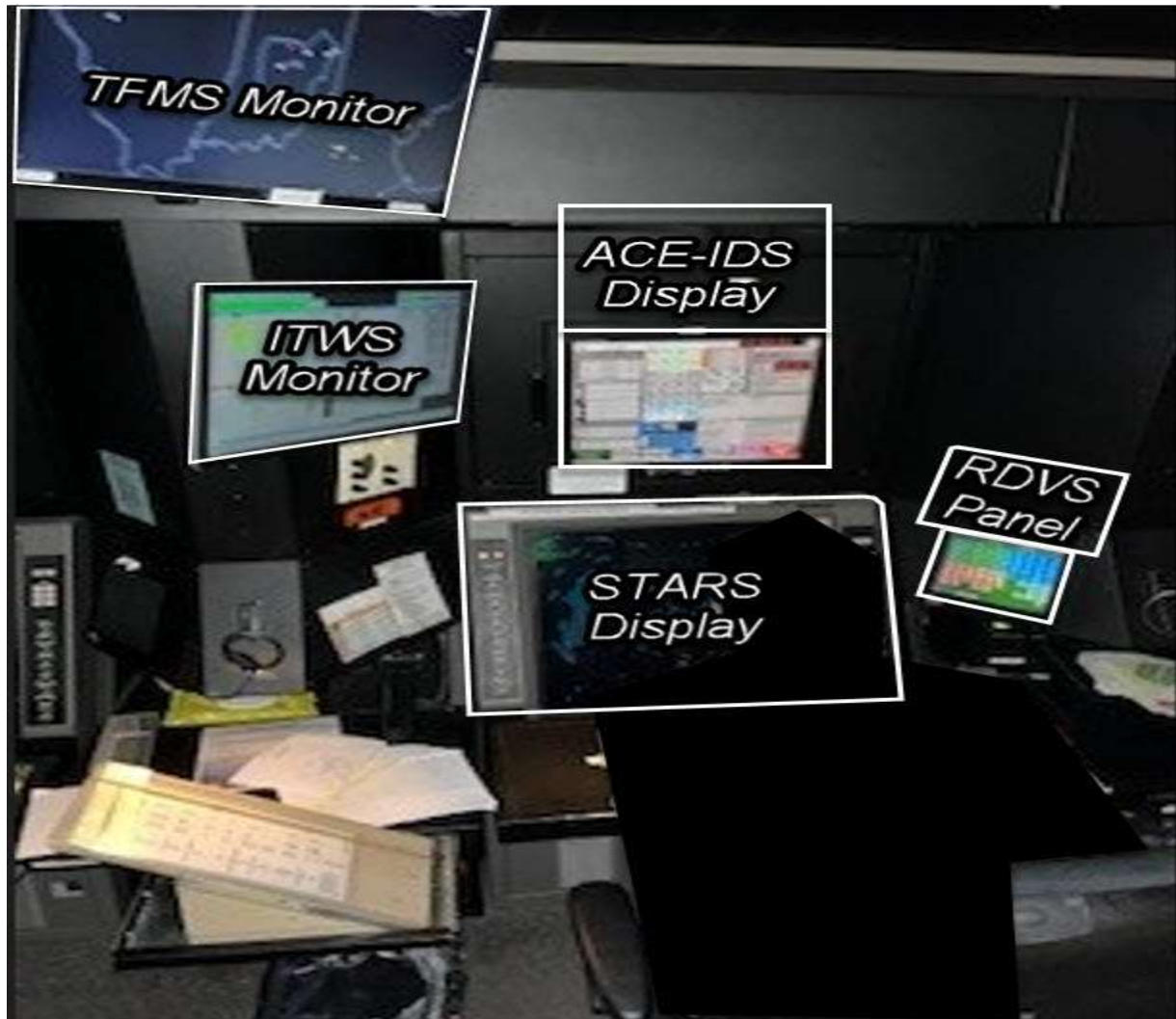
Figure 13. View of the DRE approach control position and its associated equipment.
