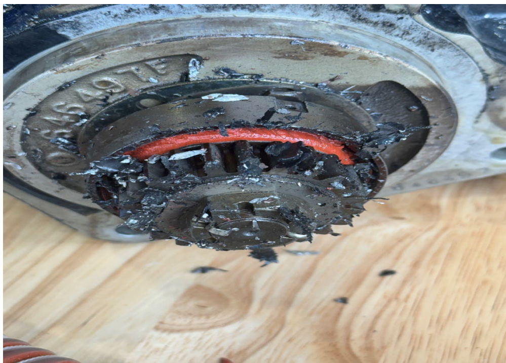
The alternator was removed and showed damage to the elastomeric bearing and large metal particles with the case.
