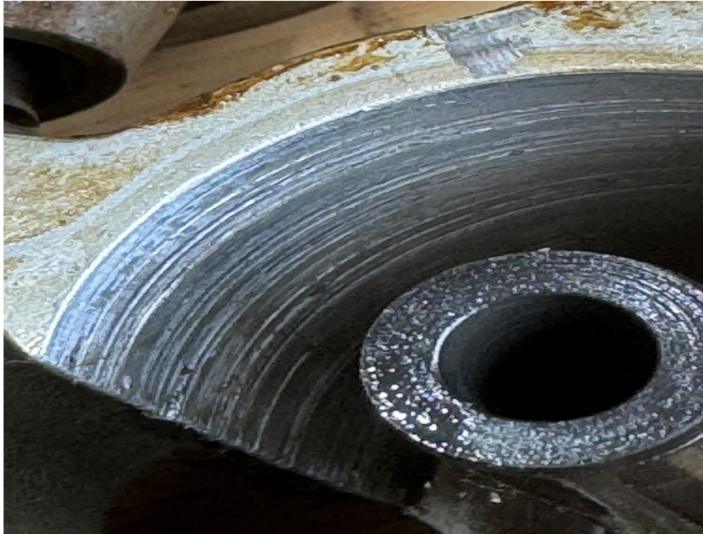
Oil pump housing showed damage to the inner walls.
