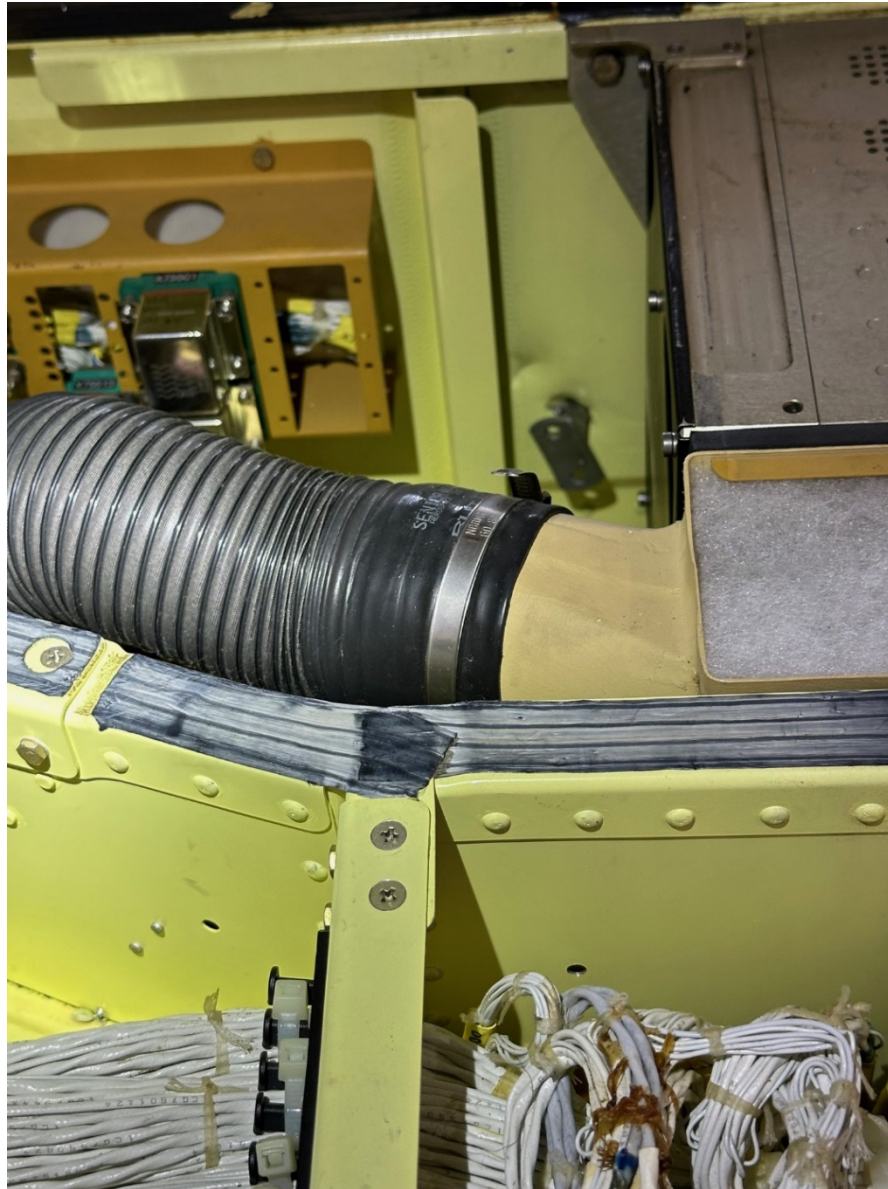
Photograph 3 - T-Bolt as found (Courtesy of Metro Aviation)
