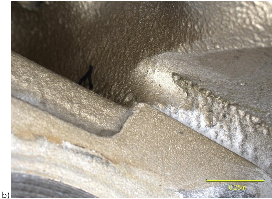
Figure 7. a) Overview image of the as received cylinder with the cracked exhaust rocker box and b) image of the blended outer edge.
