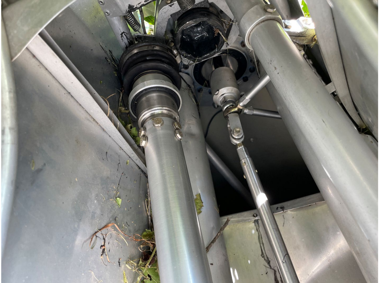
Figure 5. Failed rotor drive coupling.
